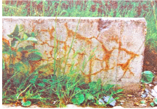
Figure 4.1: Map cracking due to ASR deterioration on a concrete wall (Stark 2008)
